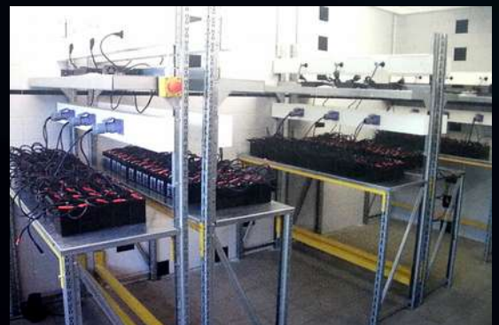
TÜV Certificated Battery Test-Room
